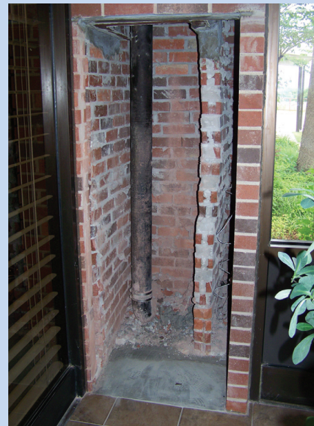
It’s not very attractive right now, but this gaping hole in the building’s front entryway will house the Pay•As•You•Go payment kiosk. It is scheduled to be installed sometime this summer.
